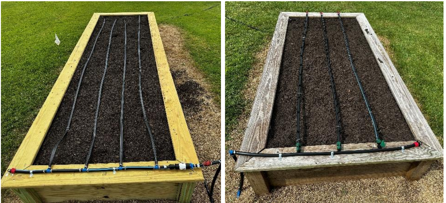
Figure 2. Example of raised bed with drip tape emitter (left) and with in-line dripper (right) installed at the Middle Tennessee Research and Education Center, University of Tennessee, Spring Hill, TN.
